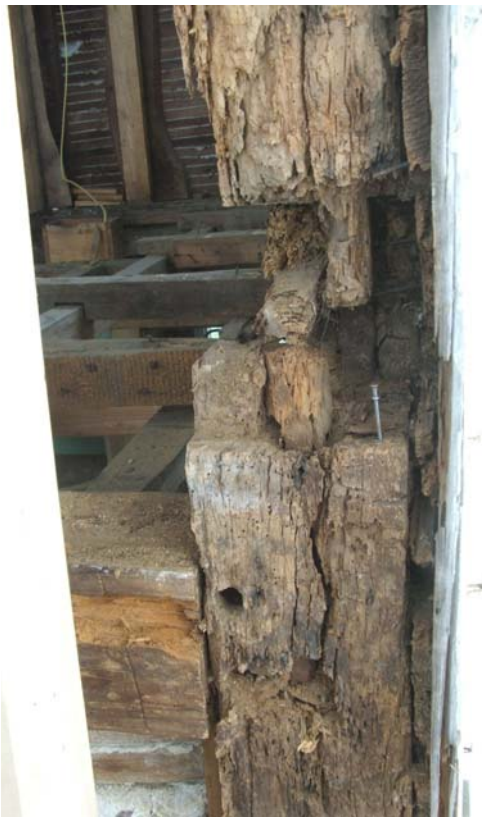
Figure 89 NW Corner Post Deteriorated Joint
