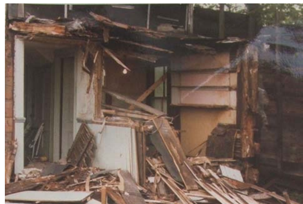
Figure 52 Barrett E. Entry shelves JW Adams 1977 East Ell entry area shows former buttery shelves and partition remains.
