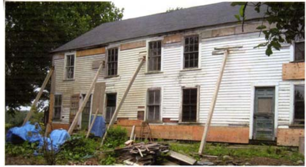
North (rear) side of Barrett House. Shows wall support structure, coverage of missing sills, and general clearing of landscape.
