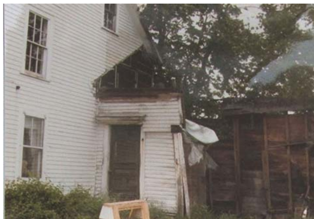
Figure 51 Barrett E Entry ruin JW Adams 1977 Photo of East Ell ruin shows rebuilt shed framing and entry details.
