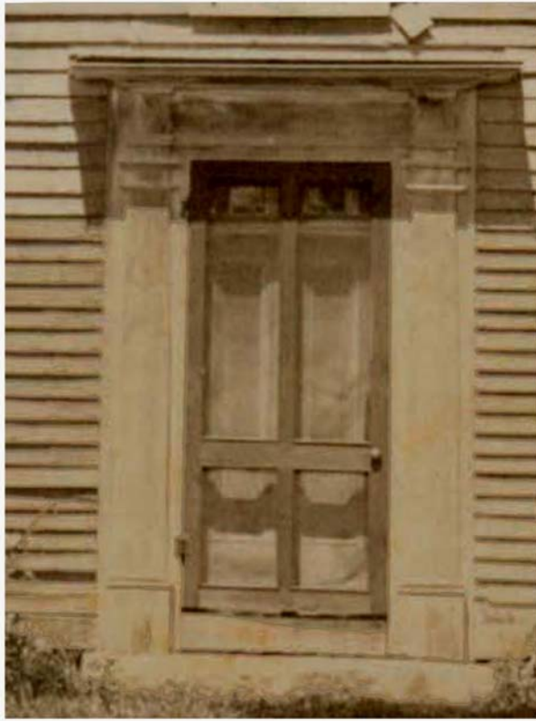
Figure 33 Barrett Main Entry c. 1880s Detail HNE The front door had pilasters and a five light transom.
