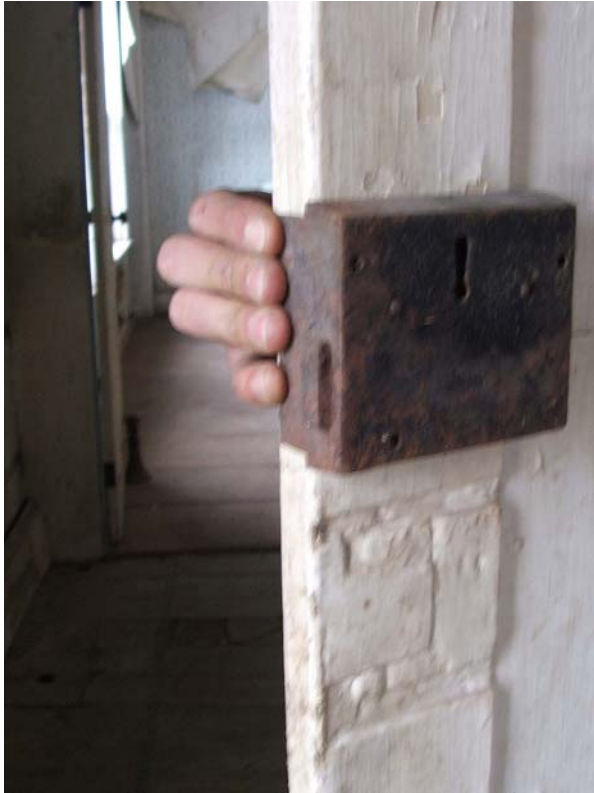
Figure 67 Muster Room Closet Lock from 2 nd floor partition
